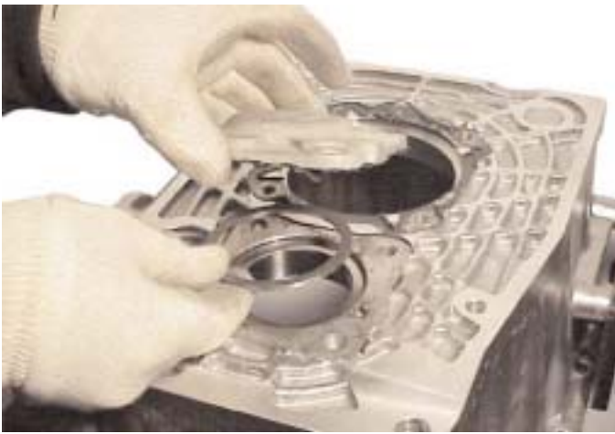
29. Invert the casing on the stand and remove the layshaft rear bearing cover and bearing spacer.
